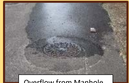
Overflow from Manhole
