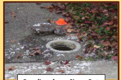
Overflow from Clean Out
